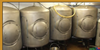
The Nook interior (above) and brewing facility (below)
